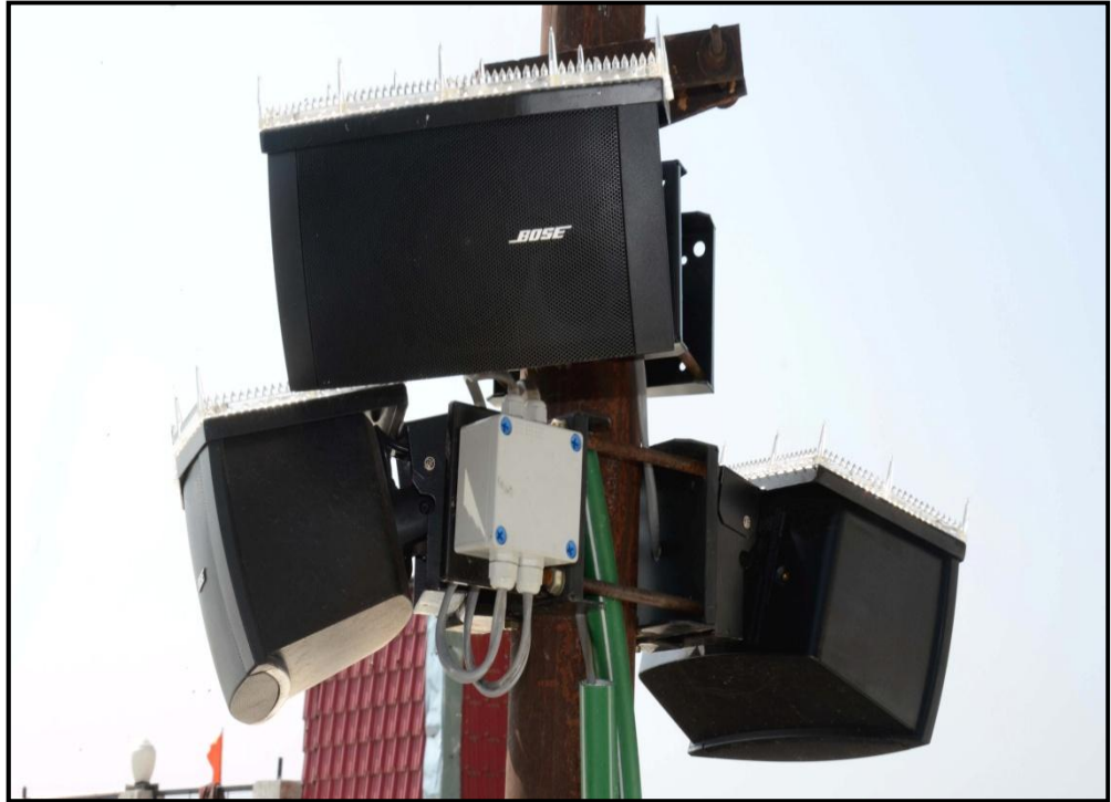
Hi-Tech Multipurpose Audio System installed on the track
