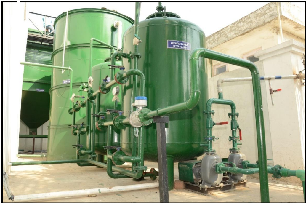
Sewage Treatment Plant at Trikuta Bhawan, Katra
