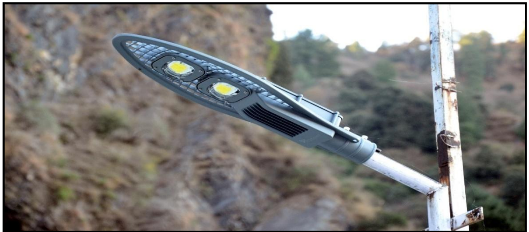
LED lights installed on the track
